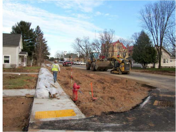
A $2.75 million street and sewer project in the town of Florence this year is one of the largest public projects in recent memory and touched 27 blocks of the community. The work included new sidewalks, replacing antiquated water and sewer mains and adding new street lights. Buy Now
